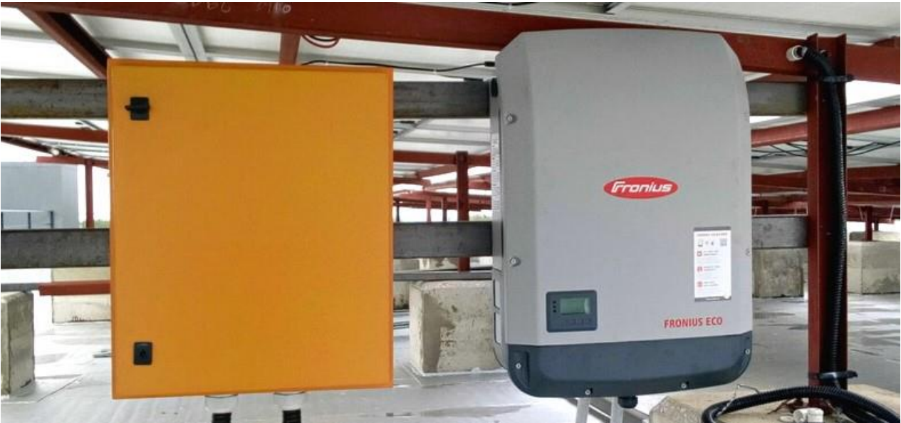
Fronius inverter and distribution box installed by us at Standard Chartered Headquarters
