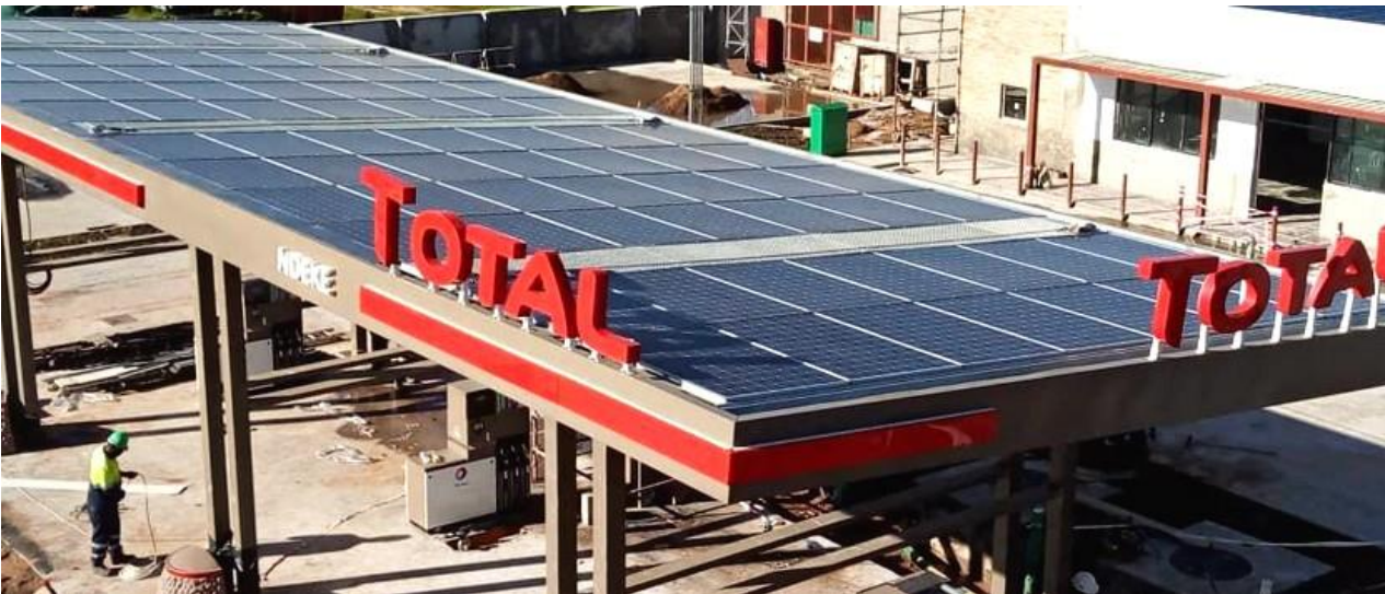
Solar panels that Techmasters installed at Total Filling Station
