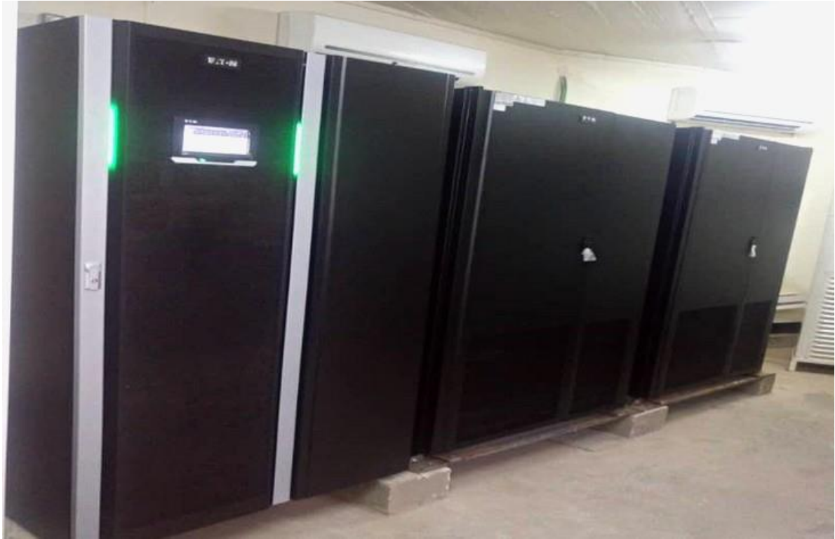
Installation of 150KVA EATON UPS and battery cabinets at Trust Merchant bank in Congo
