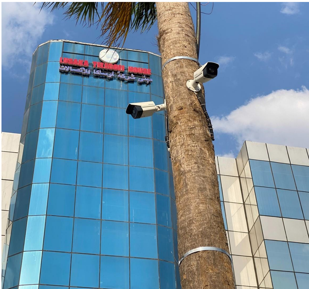
(Our CCTV Installation done at Lusaka Telecom Head Office)
