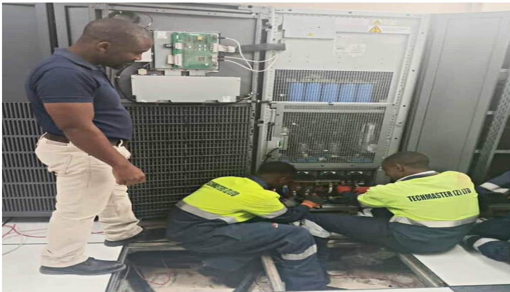
Installation of a raised floor in the ZESCO Head Office Server room.
